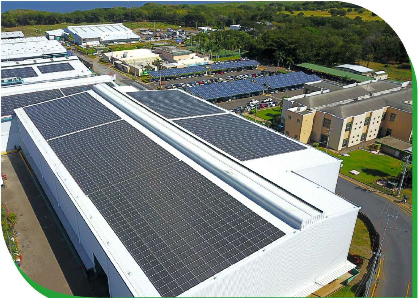
Paneles solares CCN
